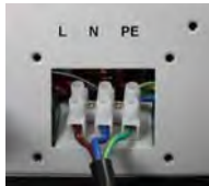
Fig. 8 AC terminals under AC terminals cover
